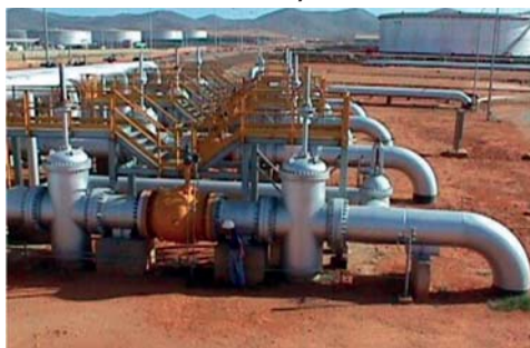
Crude Blender with remote control valves
