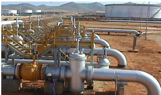
Crude Blender with remote control valves
