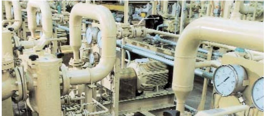
Diesel forwarding system
